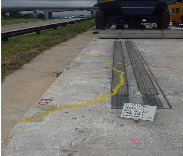
Figure 2. Crack pattern at the end of the test on the undowelled dolerite section
