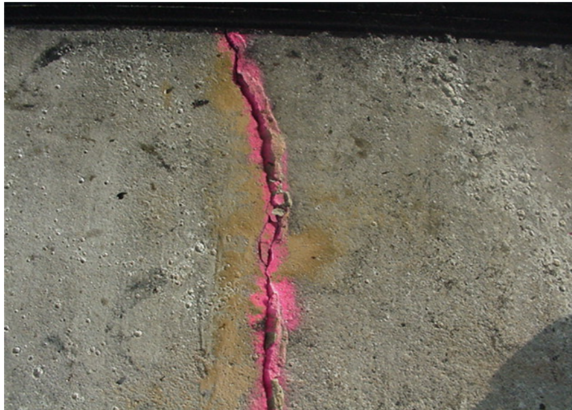
Figure 4. Spalling of a crack as a result of relative vertical movement and pumping
