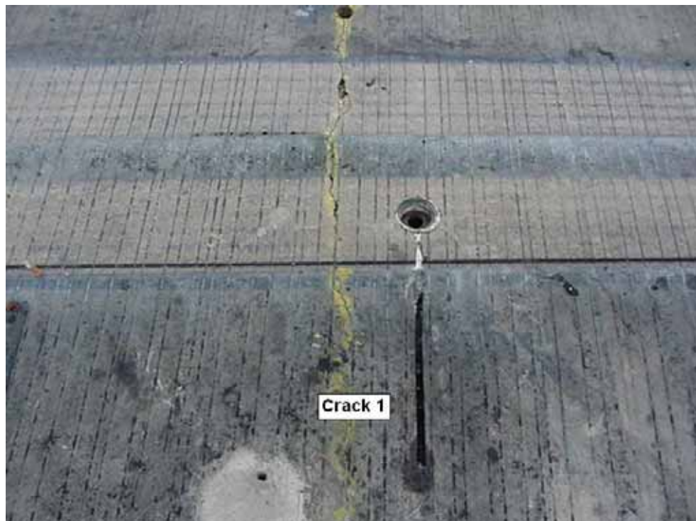
Picture 5.7: Final condition of Crack 1
