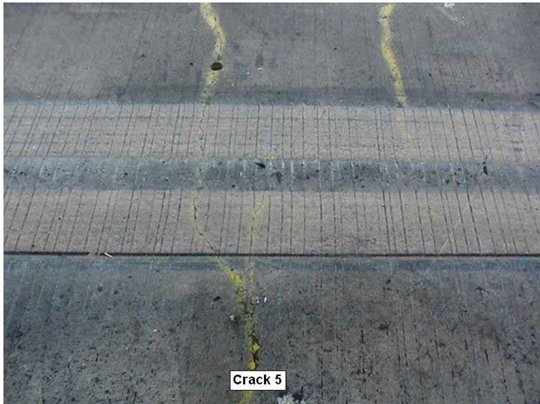
Picture 5.10: Final condition of Crack 5
