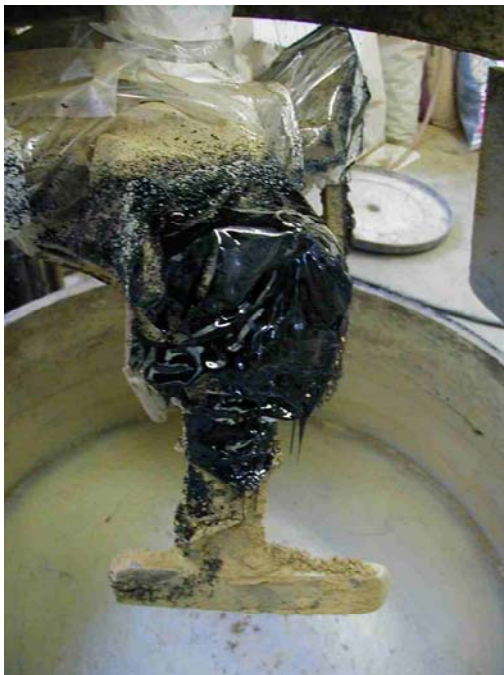
Figure 2. Mixer Arm with Bitumen
