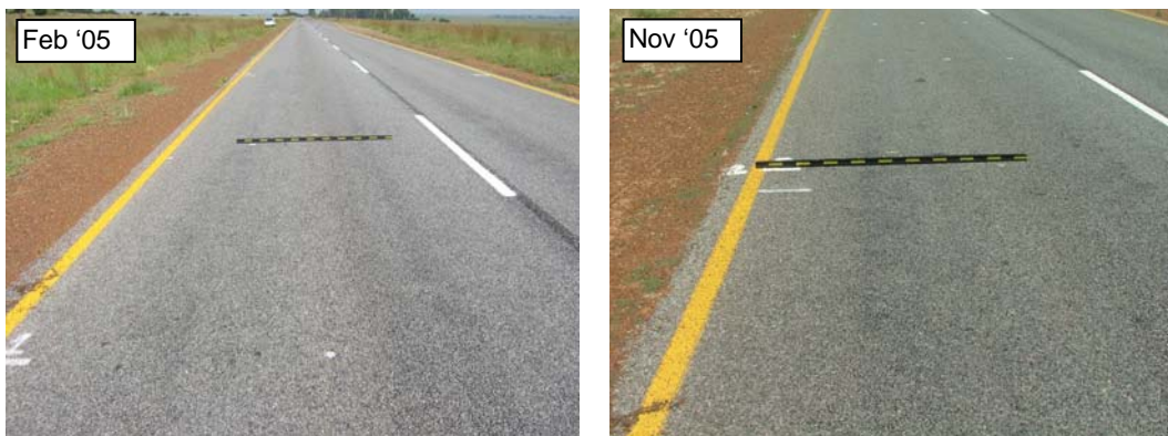
Figure 5.1: Slight bleeding in wheel paths on H3-04-G-243, Feb and Nov'05
